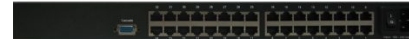
Close up of the Rear View of Cat-6 KVM showing Qty 32 RJ45 interface Ports
